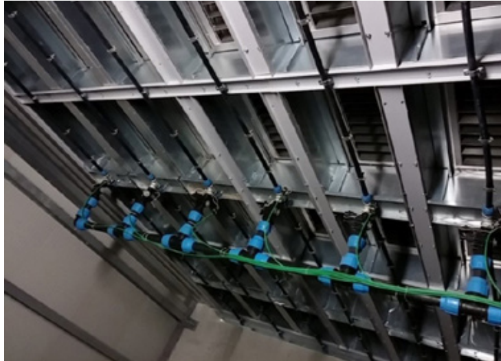
Illustration 7 - Picture of electrostatic filters of an Air Cleaning System
